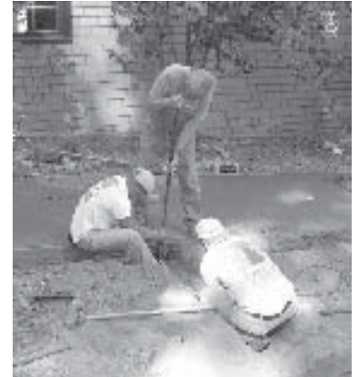
Above: Chris Elliott and Aqua Green crew members Juan and Jose work on the irrigation system.
